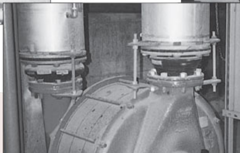
Concentric reducers installed in the suction and discharge air connections of a positive displacement high pressure blower, reduce stress to the flanges and facilitate hook-ups.
