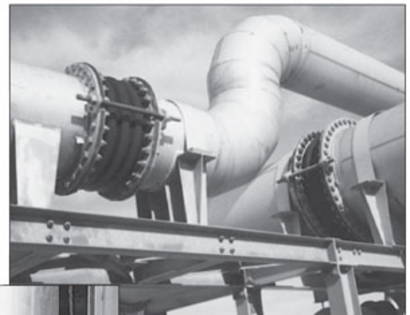
Round duct connectors installed in the duct work of a sewage treatment plant allow for major hot duct expansion.
