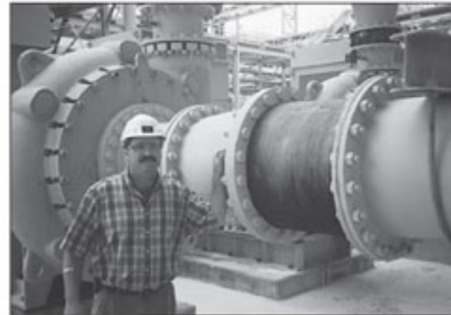
A 40" (1016mm) diameter series 100 hose installed in the suction line, drawing river water into condenser cooling service.
